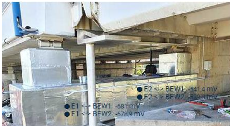
Figure 6: Galvanic cathodic corrosion protection system with zink hydrogel foil for prevention of corrosion reinforcement - Detail of the dashboard with electric potential between reinforcement and electrodes.
